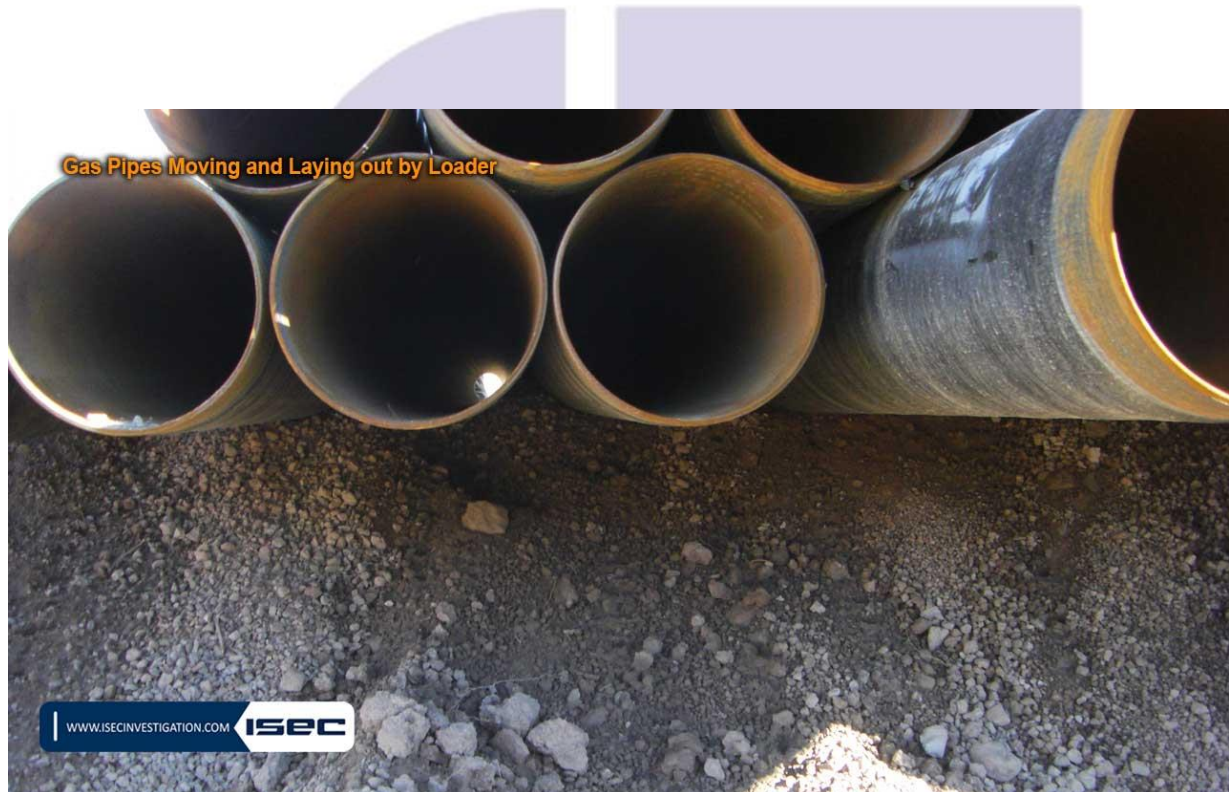
Figure 1. Smoothing and reshaping under the pipes was not made properly
